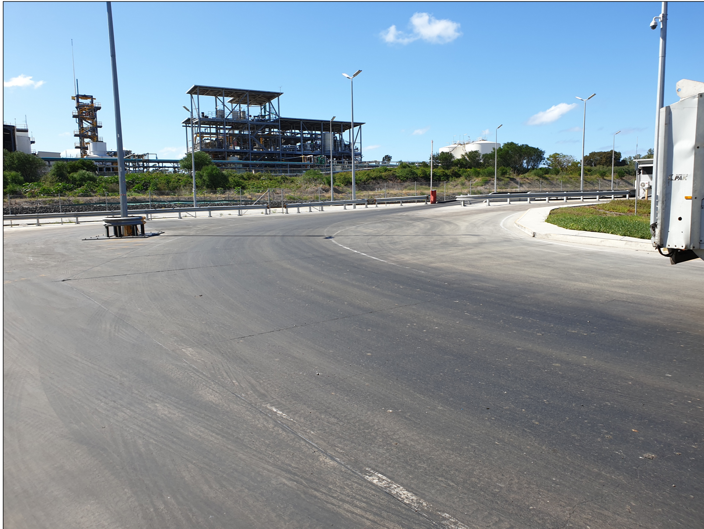
Photo 6 – A view of the BTT Facility truck entry road as found on 10 May 2019
