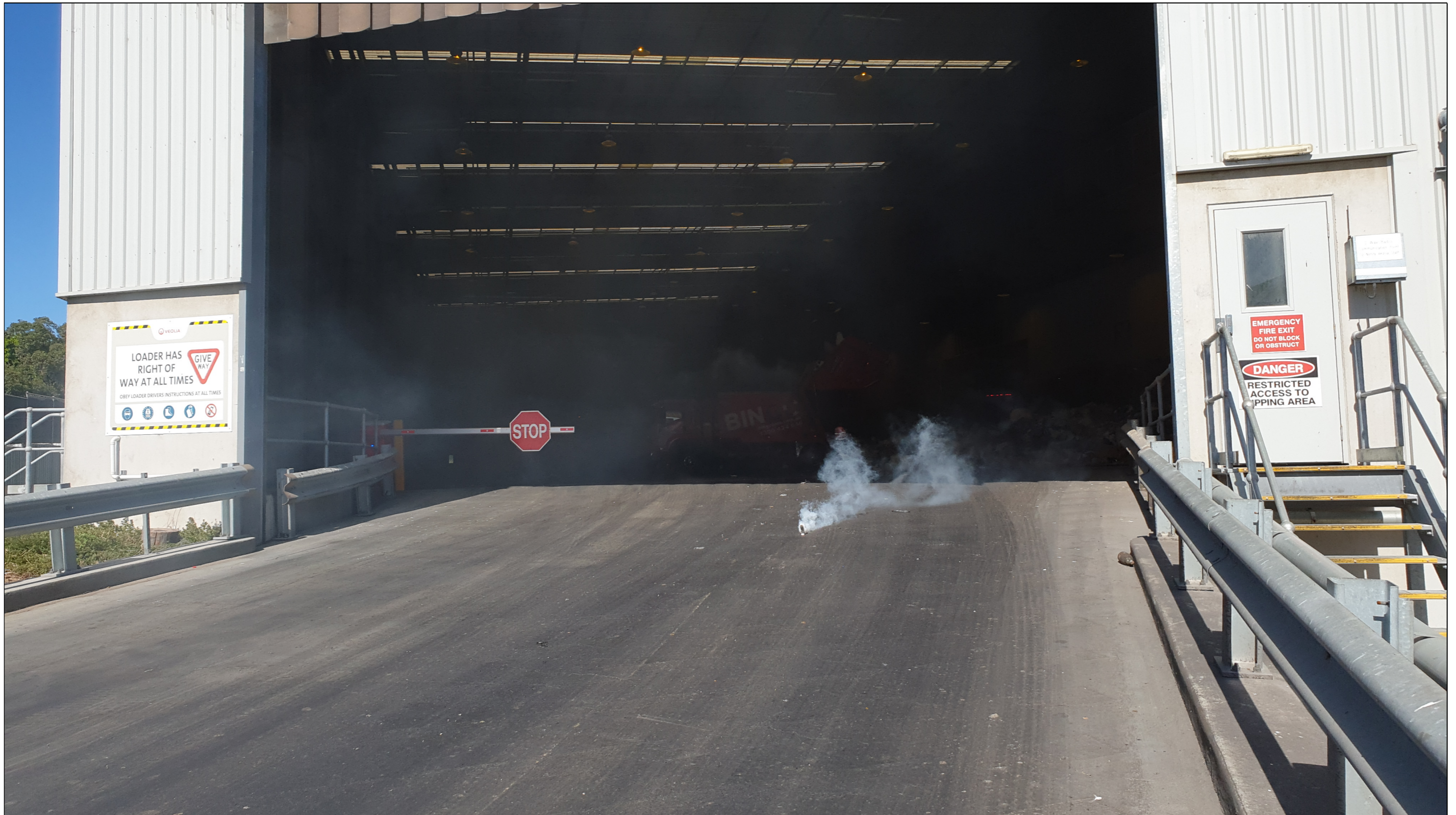
Photo 2 – Smoke testing at the truck entry point of the BTT Facility building enclosure as occurred on 10 April 2019
