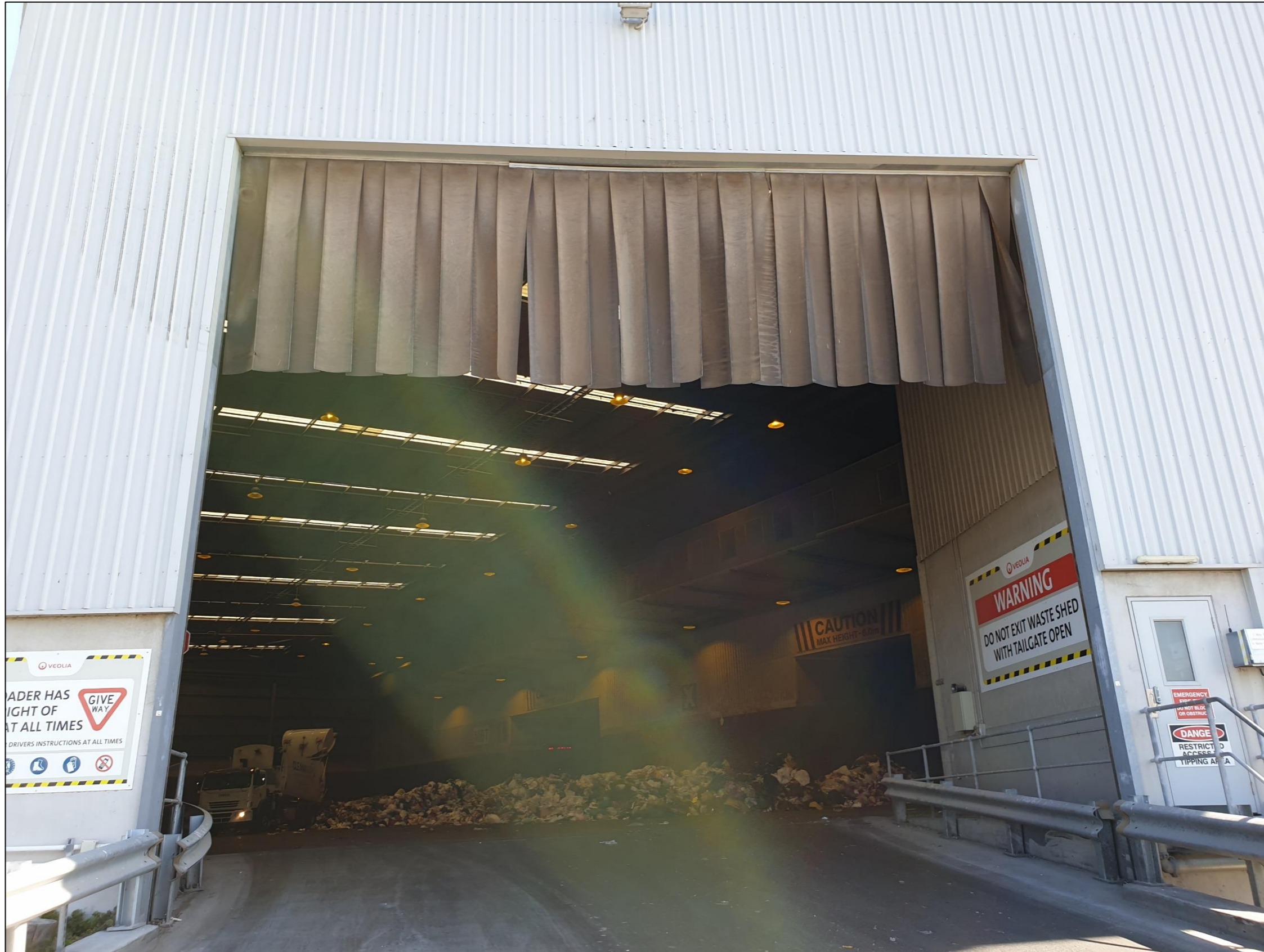
Photo 6 – A picture of the BTT Facility truck entry point as found on 2 October 2019. Note: The truck entrance plastics strips were found to be in good condition
