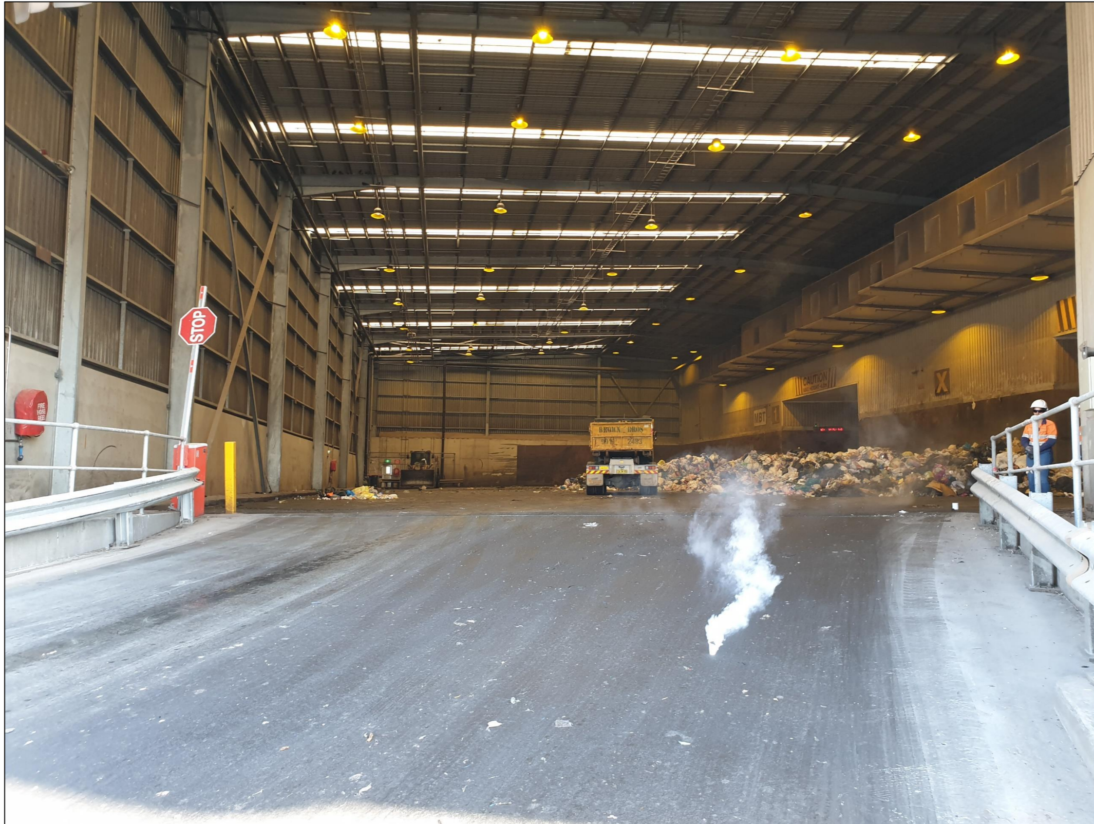
Photo 2 – Smoke testing at the truck entry point of the BTT Facility building enclosure as occurred on 2 October 2019
