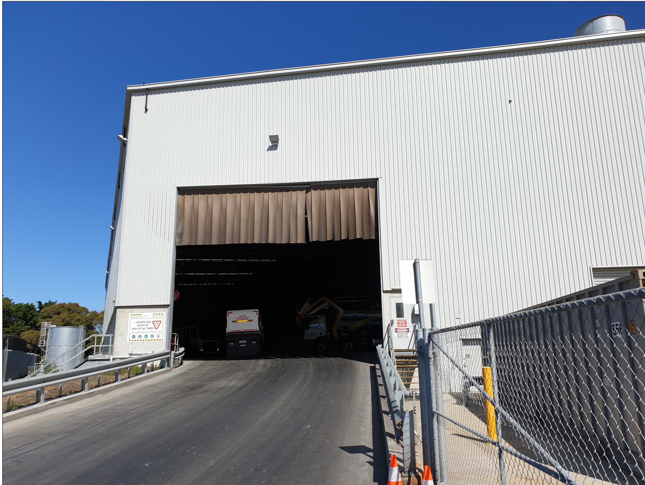
Photo 5 – A view of the BTT Facility truck entry point as found on 10 April 2019. Note: The truck entrance plastics strips were found to be in good condition.
