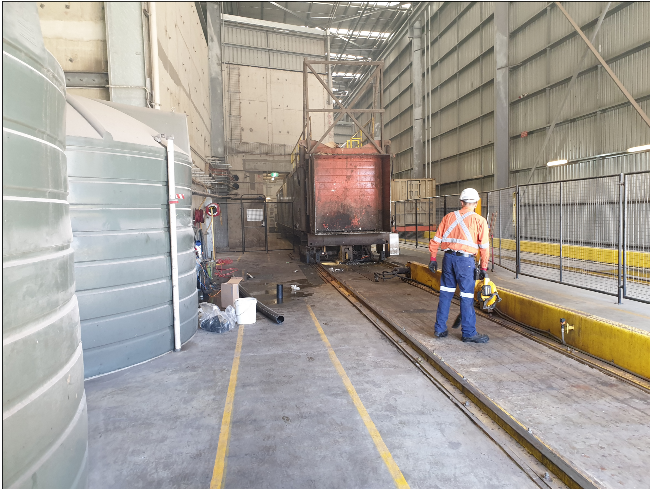
Photo 4 – A view of the BTT Facility compactor area as found on 10 April 2019
