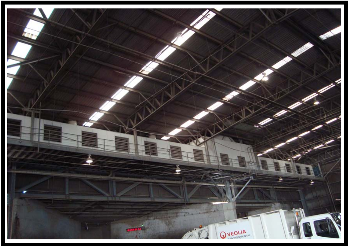
Photo 3: Newly commissioned forced air ventilation system
