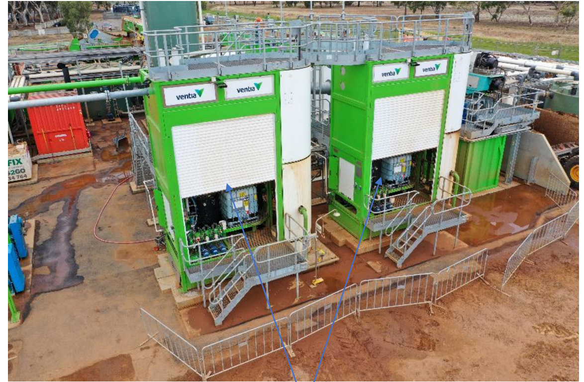
Flocculant/Coagulant Dosing Delivery Station
