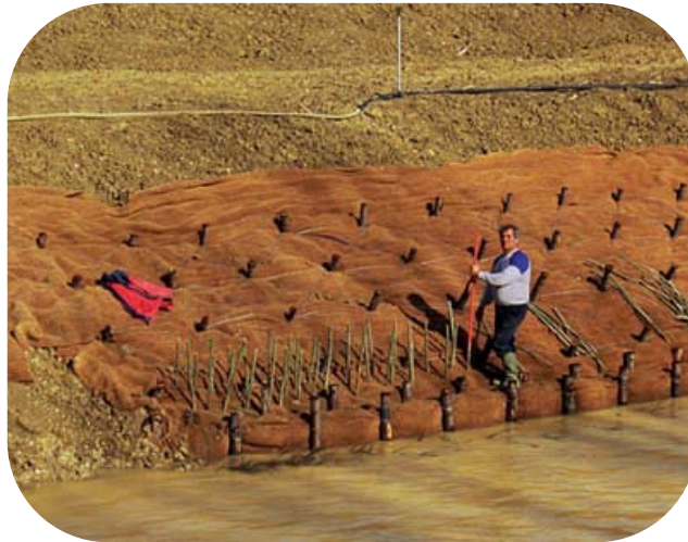
Environmental engineering in the management of riparian buffer zones
